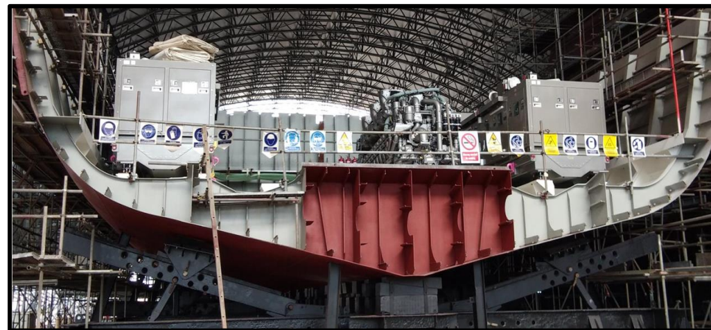
Main equipment installed before block joining
